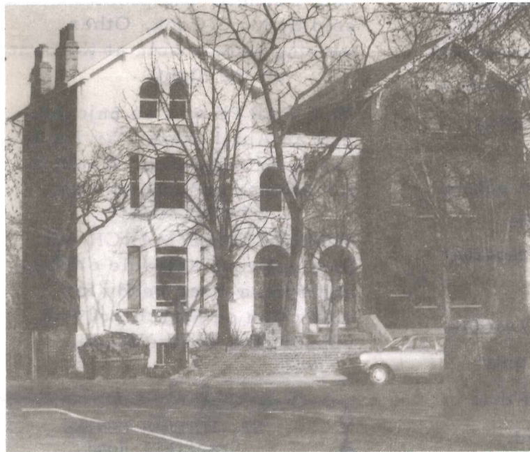
GREAT IMPROVEMENT No 6 58 Wickham Road now completed was the first property bought by Lewisham Council under a compulsory purchase order. No 56 (on right) being started.
