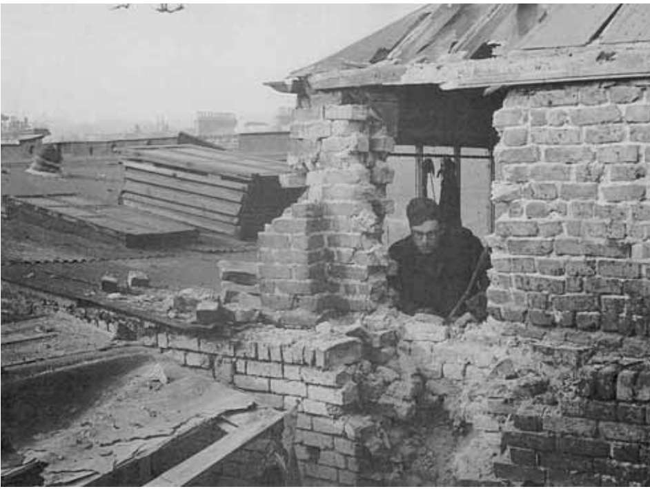
An unexploded 50kg phosphorus bomb went through the side wall of Horn's Camera Mart into the back garden of 13 Harefield Road. Captain Brooks of the Bomb Disposal Squad inspects. 8/3/1944
